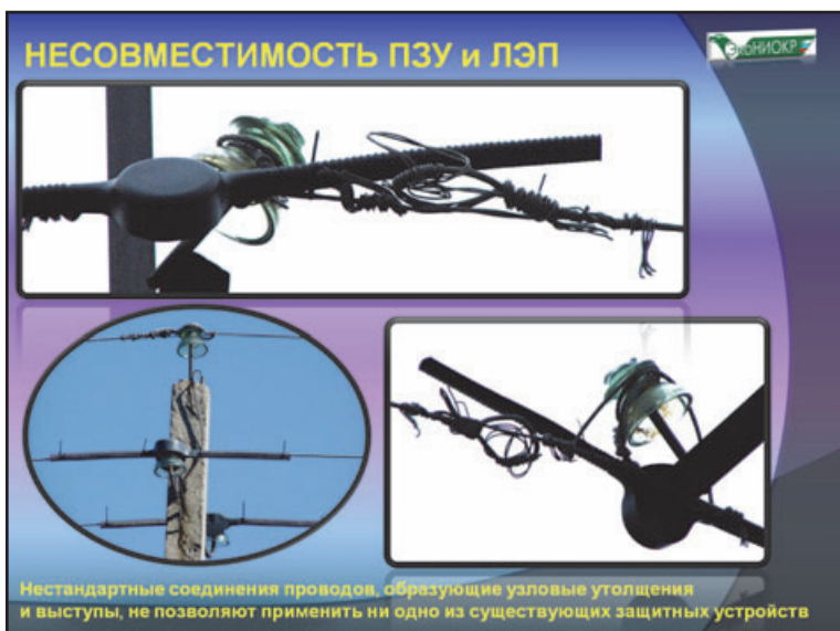
Fig. 13. Deficient BPD on a pole.
