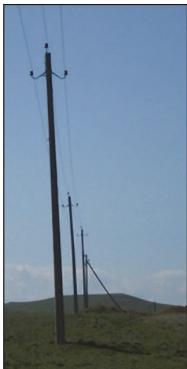
Fig. 4. Power lines in the Derbent district suspended by reinforced concrete poles.
